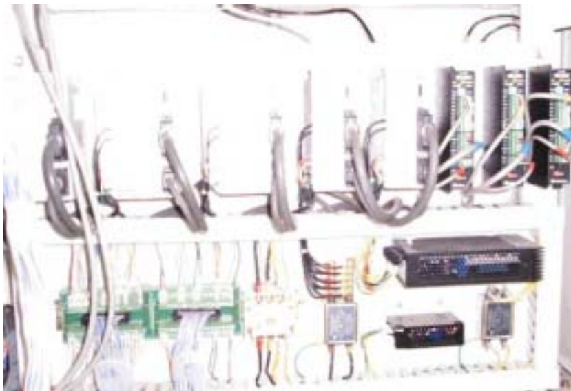
Fig.<3-17> Motor controller
