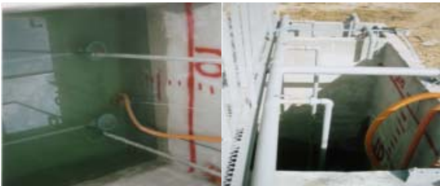
Figure 3-1-3. Photographs of treatment system
