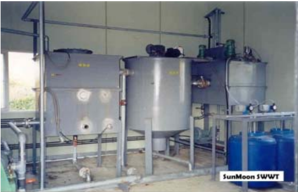
Figure 3-42. Front part of two-stage ASBF system (From right, reaction tank with 2 chemical tanks with pumps, sedimentation tank, heater exchanger)
