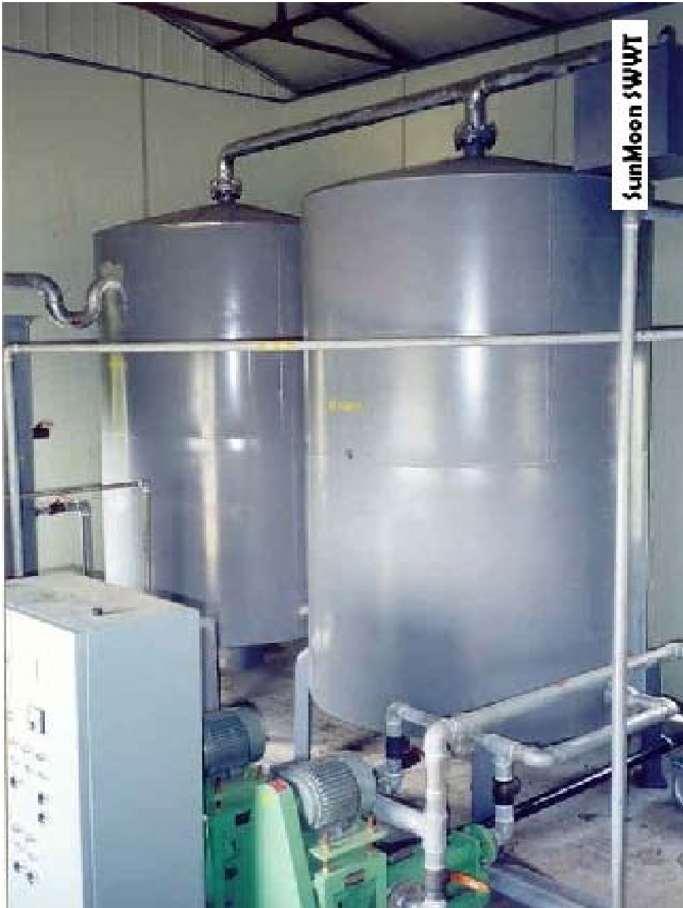
Figure 3-44. Two-stage ASBF bioreactors with two mono pumps and control system
