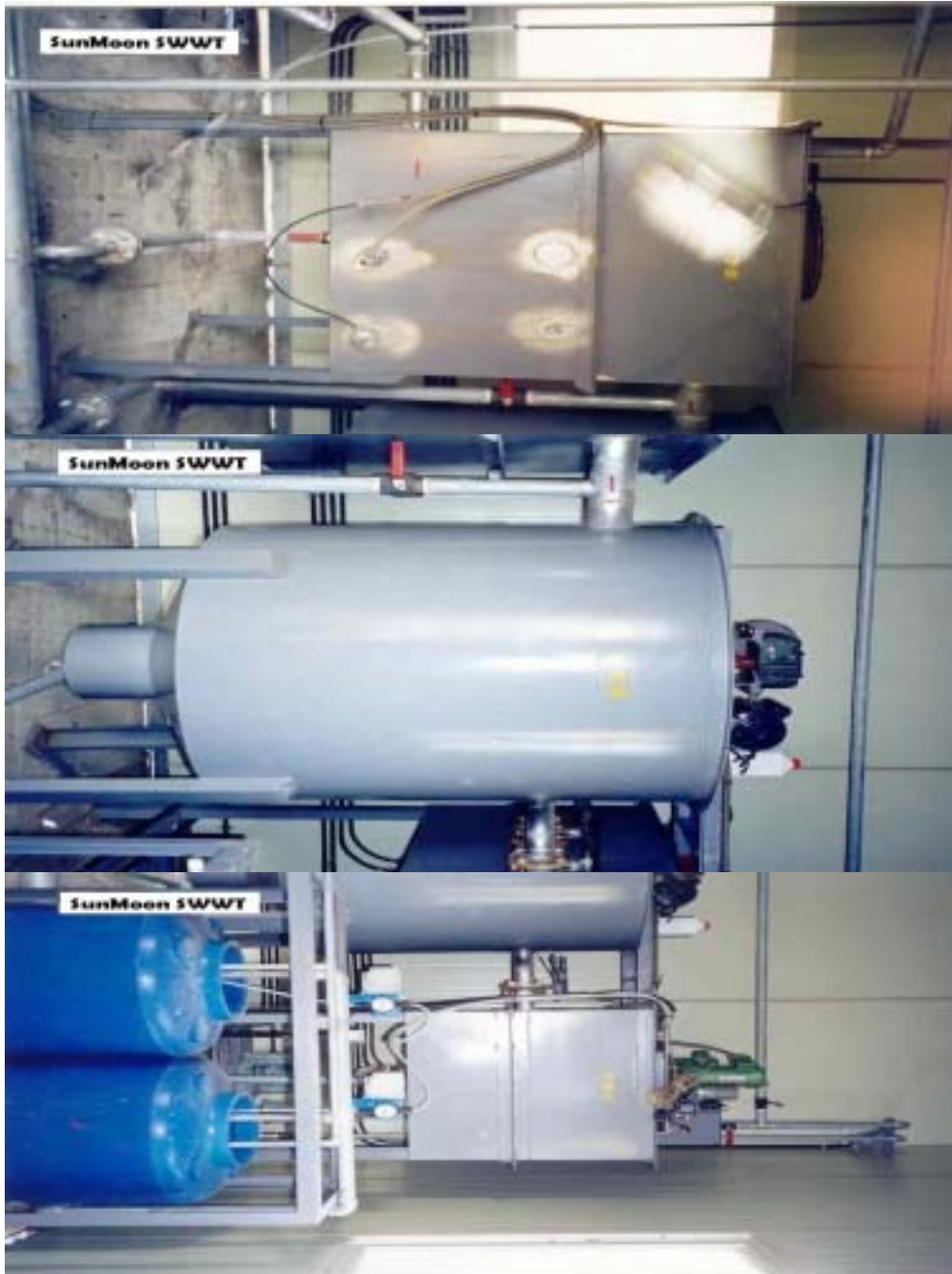
Figure 3-43. Detailed pictures of front part of two-stage ASBF system (From bottom to top : reaction tank with two chemical tanks with pump, sedimentation tank, and pre heater tank)
