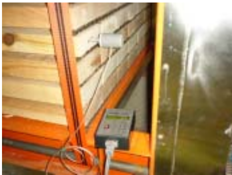
Fig. 3-5. Moisture content sensor inserted in the stack.
