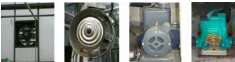
Fig. 5.14 On/off control equipments
