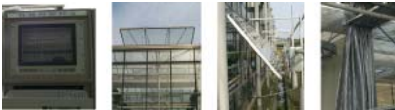
Fig. 5.13 Greenhouse control computer and open/close control equipments
