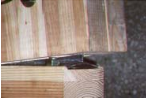
a) Deformation of hanger joint
