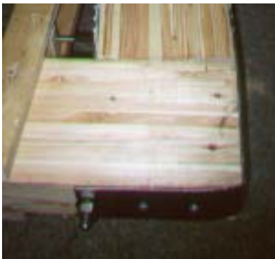
a) Failure of wood under steel plate
