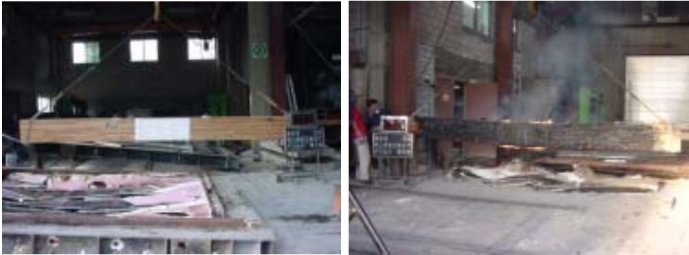
Figure 3-86. Picture of glulam beam with bolted steel gusset plate joint covered by thick(1.2mm) coating of fire-resistant paint at center.
