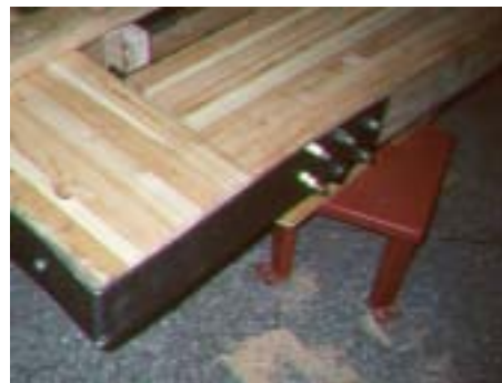
b) Deformation of steel plate
