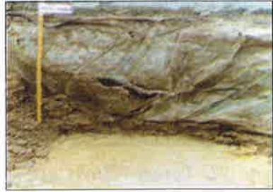
Photo 22. Planting hole of damaged street tree.
