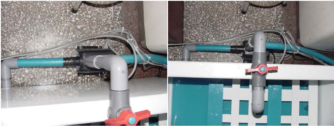
Fig. 2-1-10. Pump used to circulation sea water.
