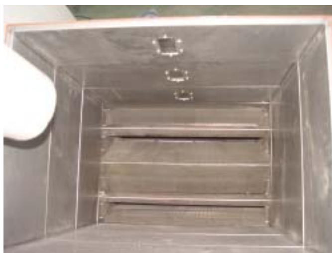
Fig. 3-17 View of the drying section.
