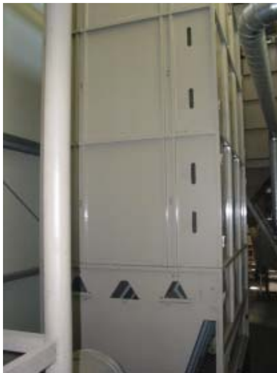
Fig. 3-63 View of circulation grain dryer.
