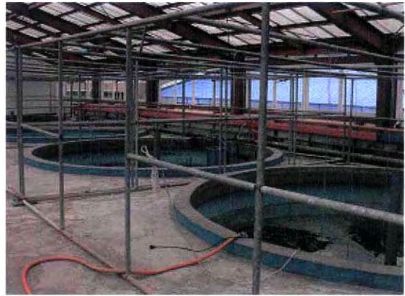
Fig. 12. Circular tanks of 28 m 2 in surface area.
