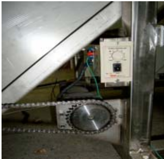
Photo. 54. Motor speed controller.
