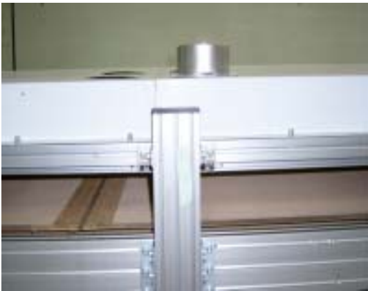
Photo. 58. The upper hole of exhaust energy duct.
