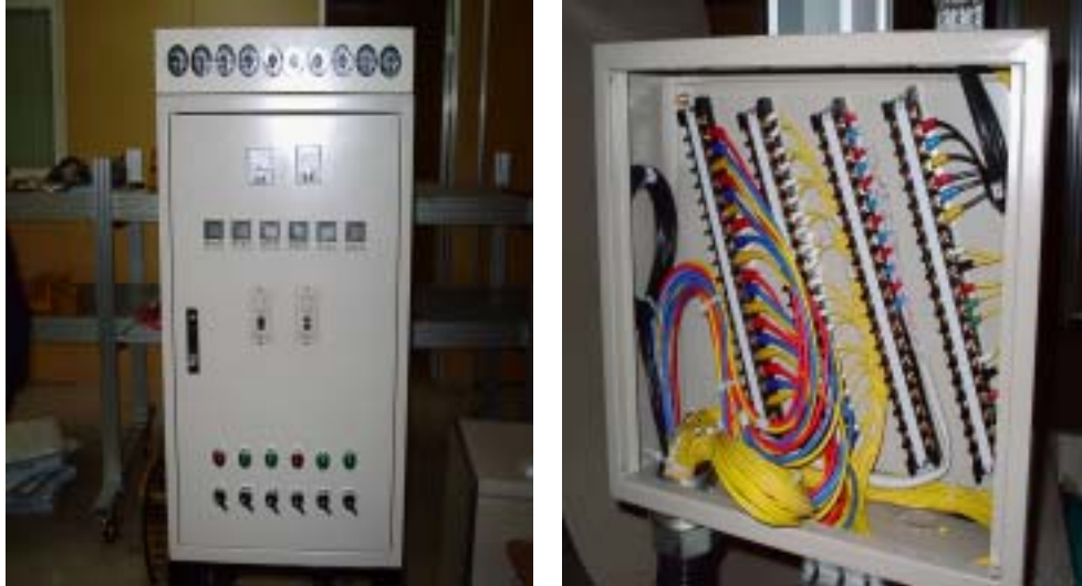
Photo. 34. Controlling board and distribution board.
