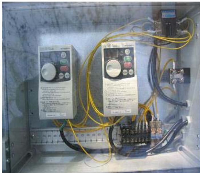
Fig. 22 Photograph of control box.
