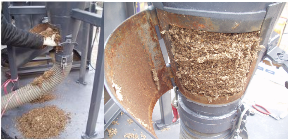
Fig. 45 Problems occurred at the outlet of cyclone on prototype
