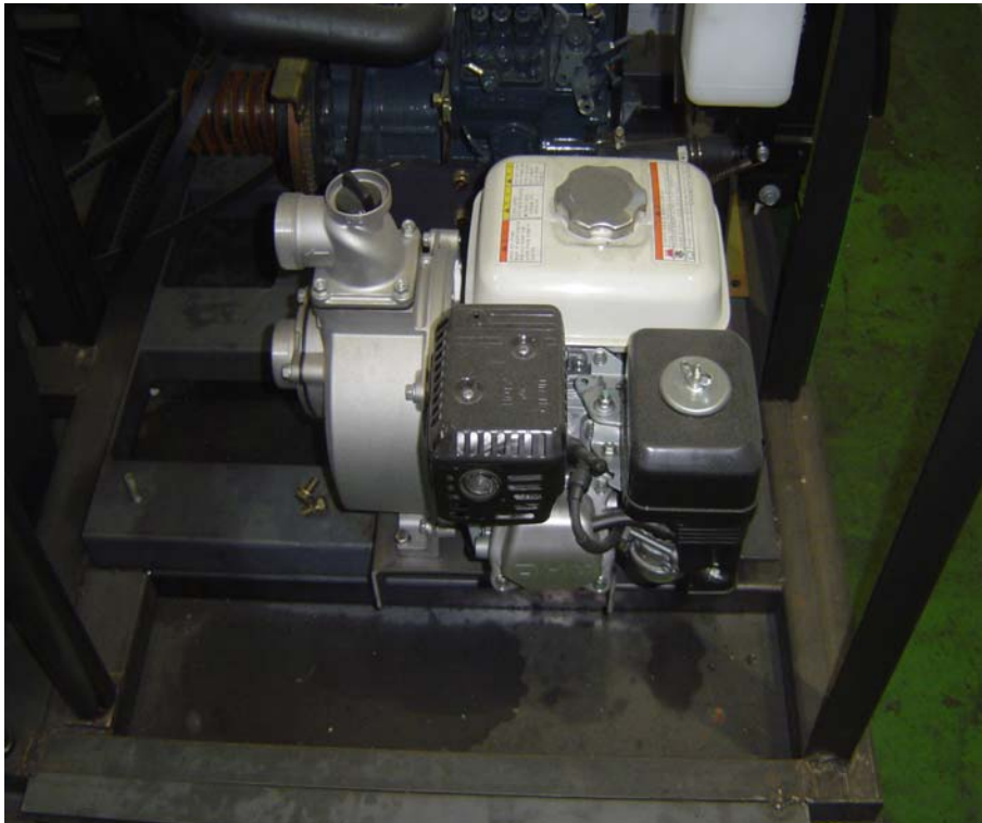
<Fig. 3-53> Water meter engine frame
