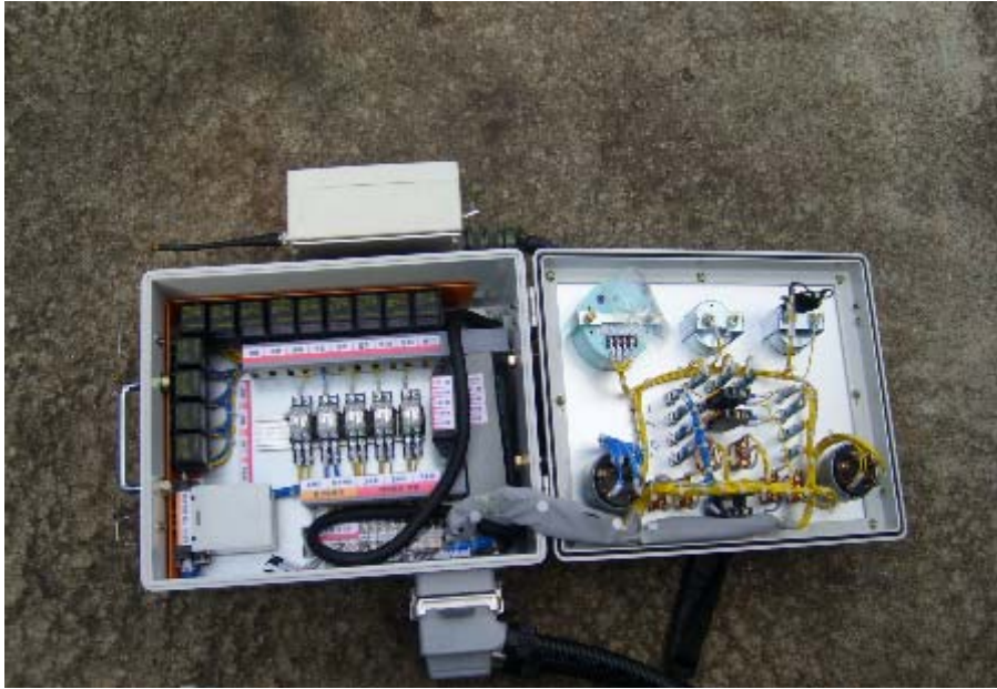
<Fig. 3-60> Inside of a radio regulator
