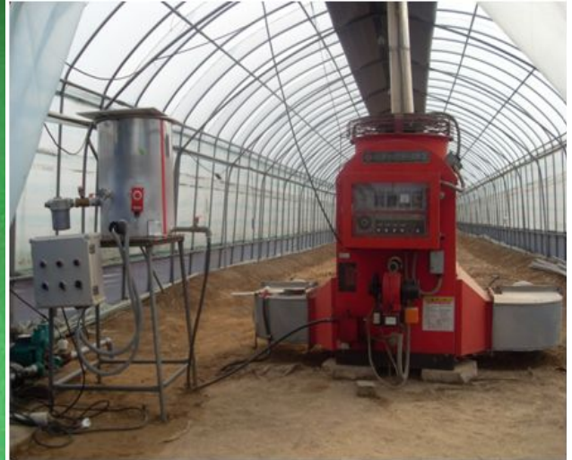
Fig. 32. Hot air heater in greenhouse
