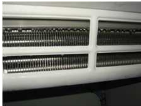
Photo 7 Evaporator fins and coil after defrost
