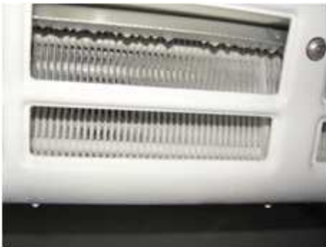
Photo 6 Evaporator fins and coils with frost formed after 4 hours operation
