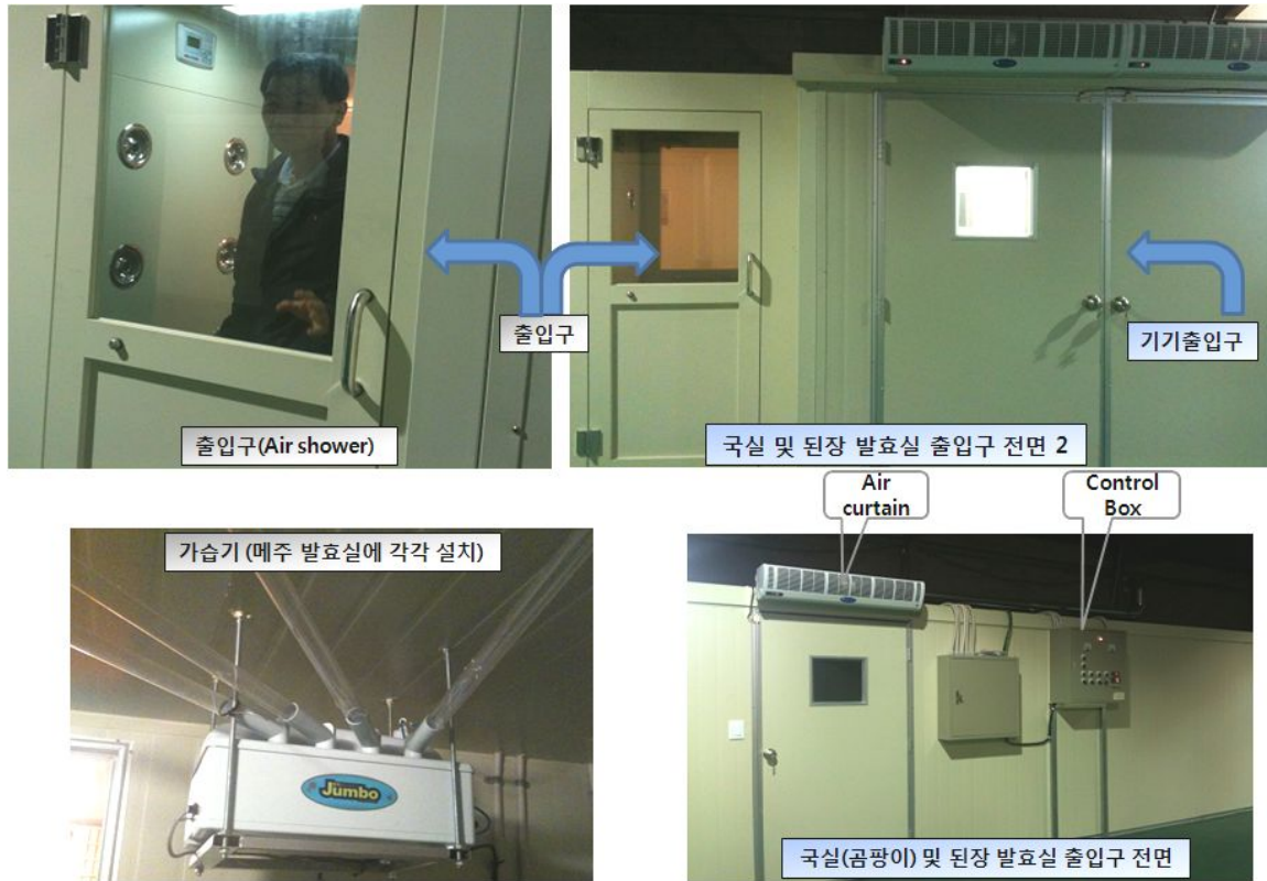
Fig. 38. Air-shower, humidifier, and temperature controller.
