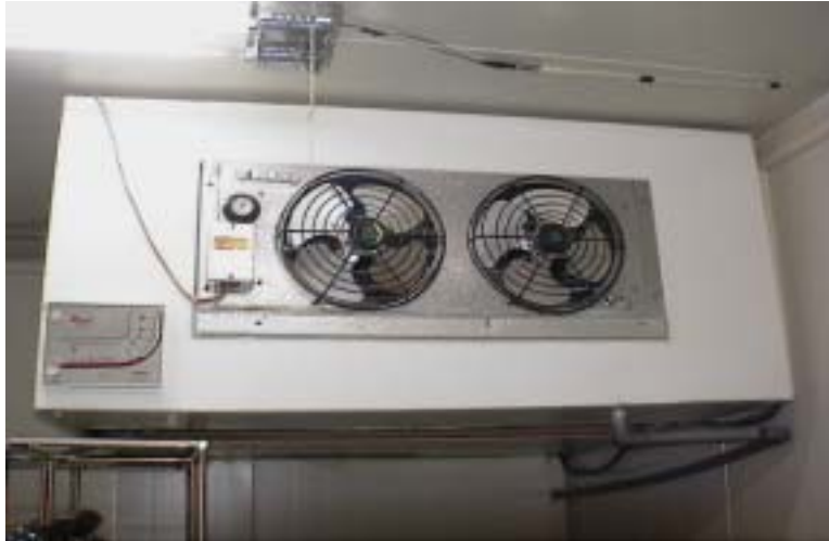
Figure 3.3.1.3 Cooling fan in the artificial growth control room
