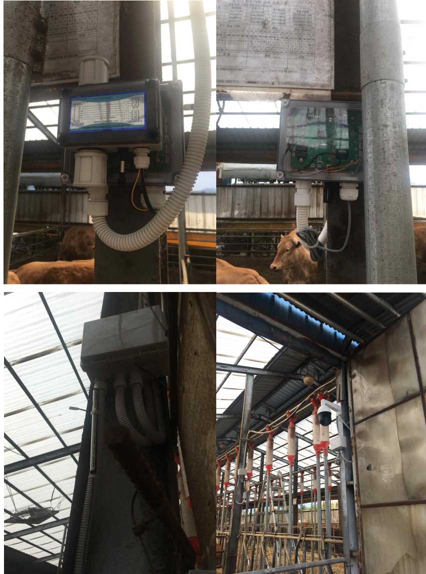
그림 1-119. Components of smart pilot farm, in order left upper; air flow, temperature & humidity, node device, P&T circuit camera
