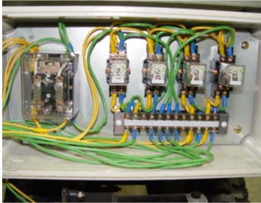
Figure 28. Photograph of the electric circuit of the control unit.
