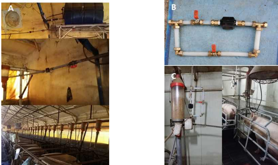
Fig. 31. Installation of magnetic equipment in pregnancy room (A), control valve (B) and parturition room (C) of experimental farm
