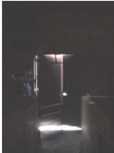
Fig. 27 A gap in a door causing inexpectant air-infiltration
