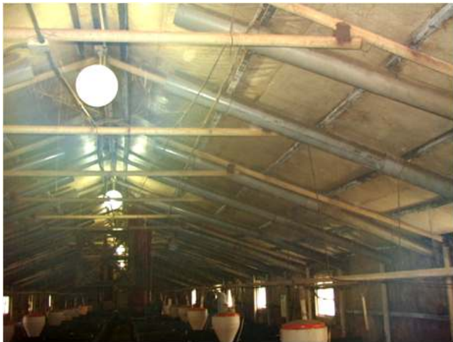
Fig. 15 Pipe inlet system at pig house A
