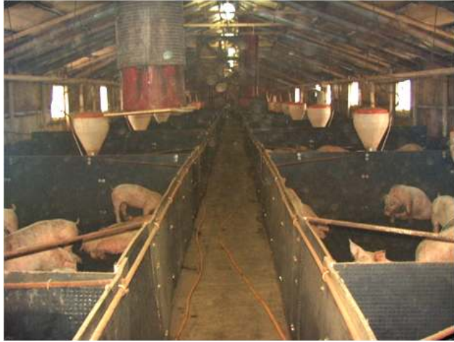
Fig. 14 Exhausting duct with fan at pig house A
