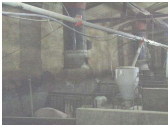
Fig. 7 Suction ducts for negative pressure ventilating system in the pig house
