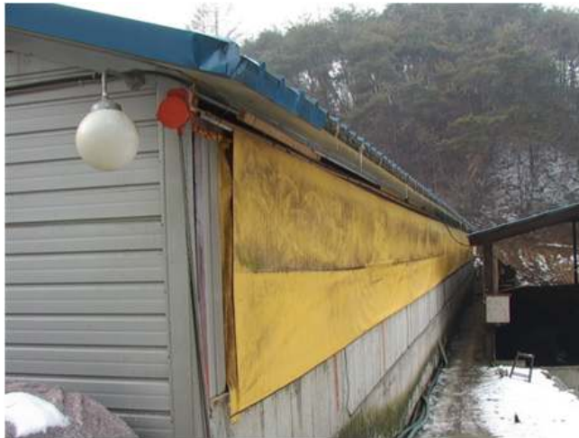
Fig. 17 Winch curtain at side wall at pig house B
