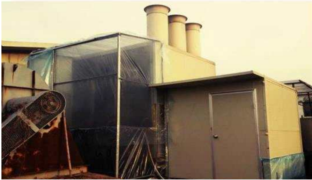
Fig. 9 Biofilter system installed at Suwon, SNU livestock farm, South Korea
