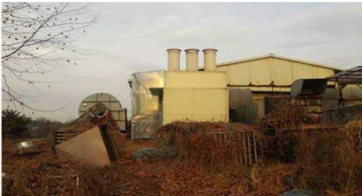
Fig. 10 Biofilter system installed at Suwon, SNU livestock farm, South Korea
