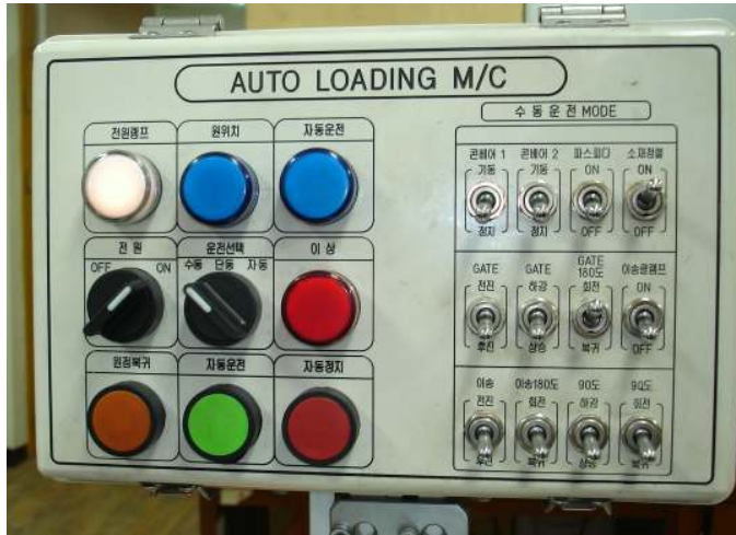
Fig 29. Control panel unit.
