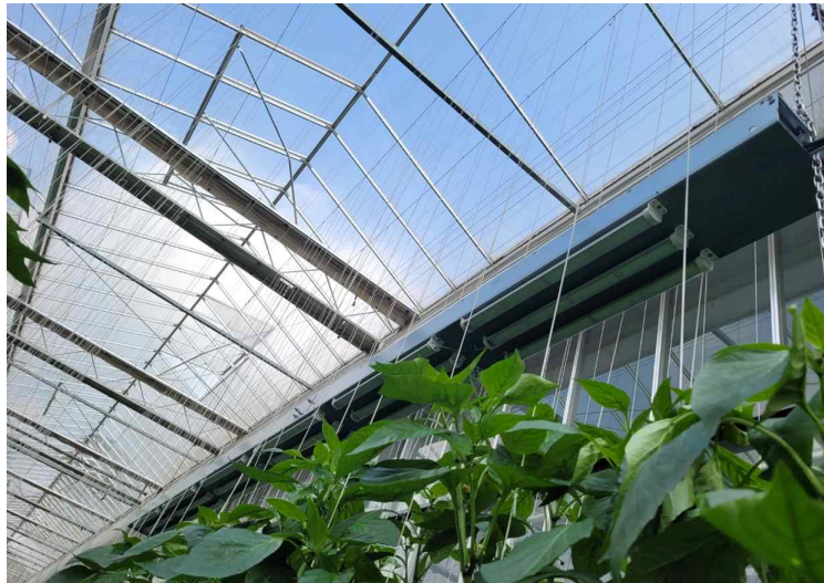
Fig. 2-28. LED lighting installed on plants.
