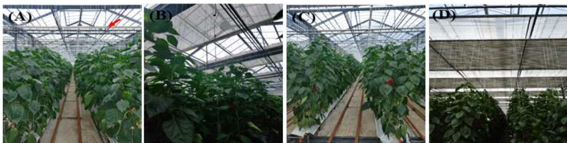
Fig. 3-30. Installed screens in the greenhouse located in Injae, Gangwon-do, South Korea. A and B is 1-layered screen, while C and D is 2-layered screen).
