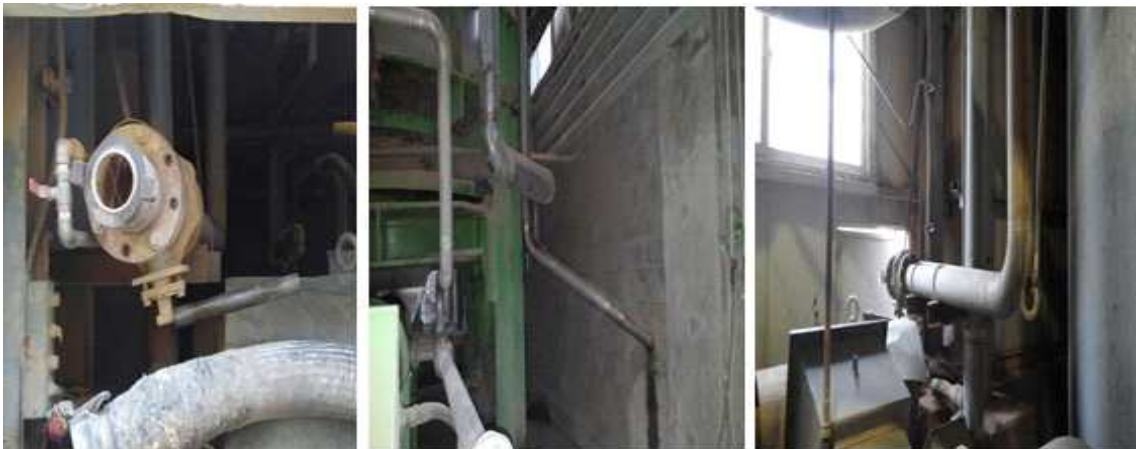
Fig. 3.196. Air blower and pipe lines to rice husk organic filler chest.
