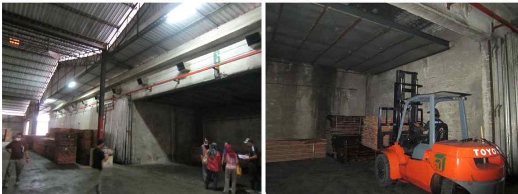
Figure 3-11. Kiln drying system for laminae in MY-D
