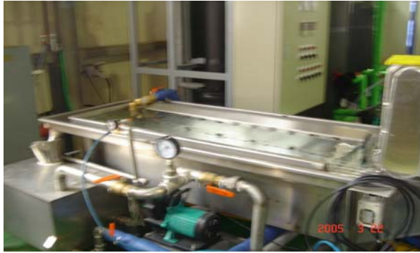
Fig. 30. Local installation of washing apparatus.
