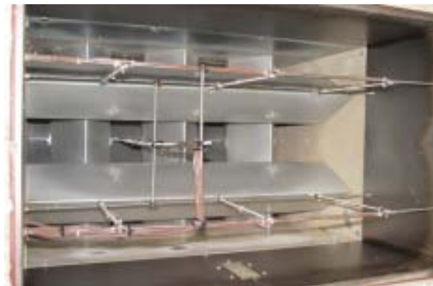
Fig. 3-33 View of air outlet.
