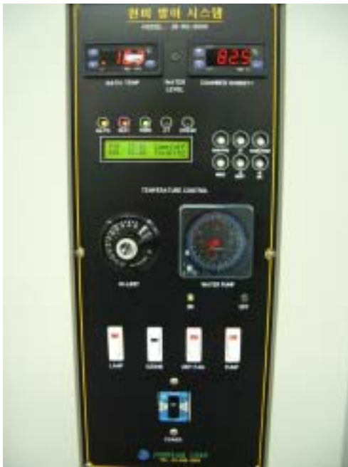
Fig.3-32 The control panel
