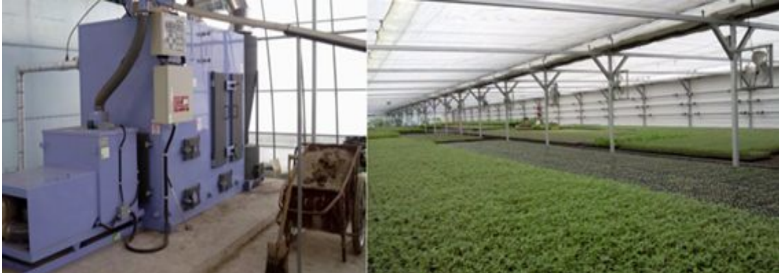
Fig. 4-3-7. Pellet boiler and green house.
