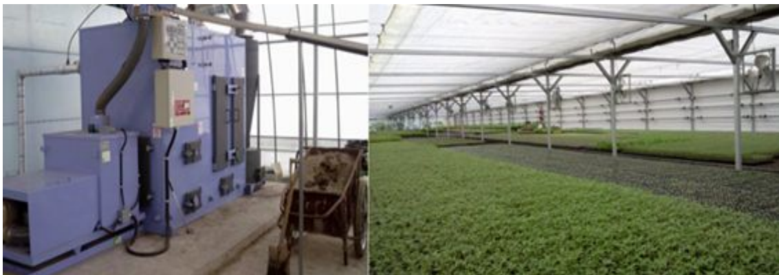
Fig. 4-2-13. Pellet boiler and green house.
