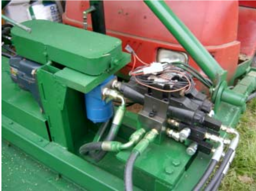
Fig. 23 Solenoid valves & hydraulic motor
