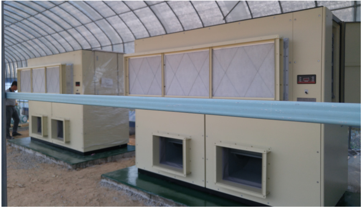
<Fan coil unit>
