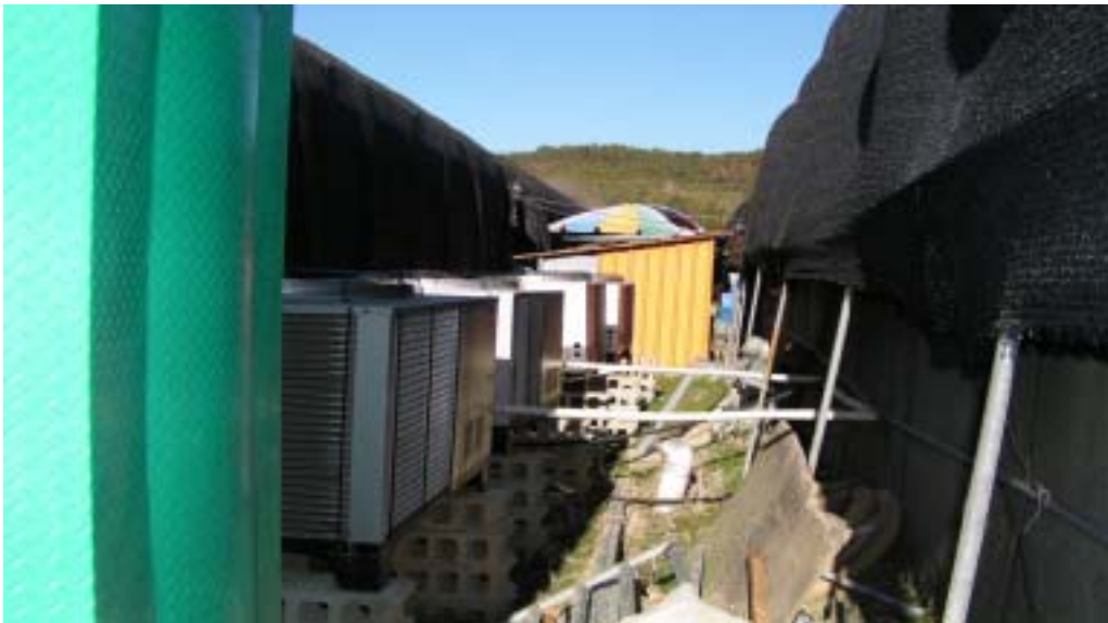
Photo 2-5. View of cooling compressors.
