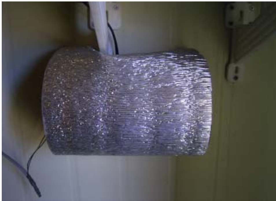
Photo 2-23. View of relative humidity sensor and fan.
