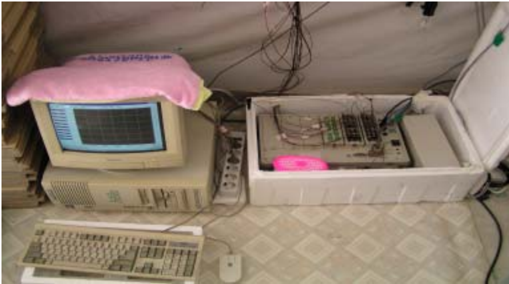
Photo 2-9. View of control panel, data logger and computer.
