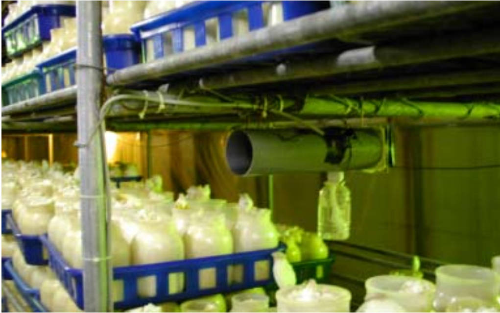
Photo 2-2. View of typical temperature instrumentation.
