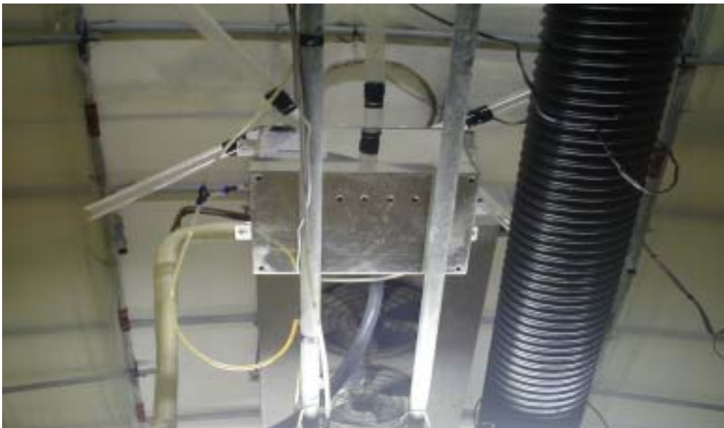
Photo 2-3. View of ultrasonic humidifier, evaporator and intake duct.
