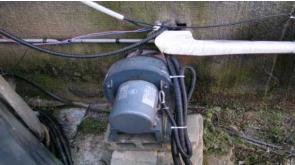
Photo 2-6. View of exhaust fan and duct.
