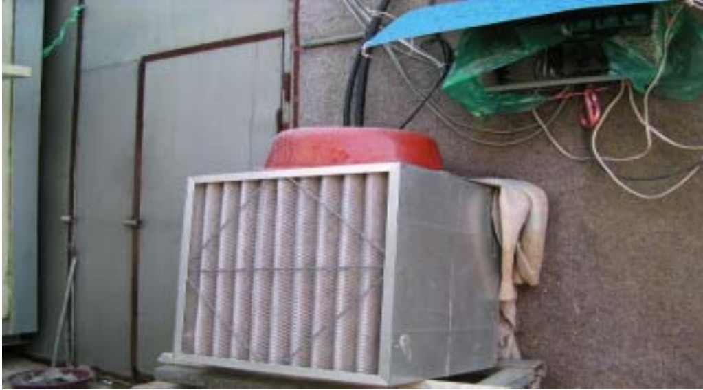
Photo 2-7. View of intake air filter.
