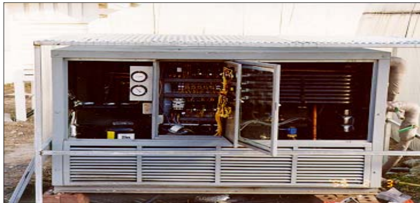
Photo 2-18. View of heat pump system.
