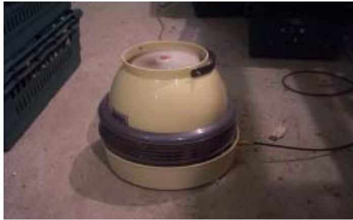
Photo 2-17. View of humidifying system.
