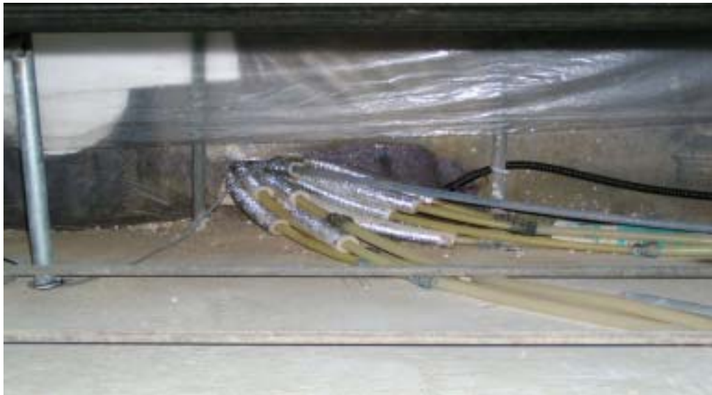
Photo 2-8. View of pipes to circulate heat water.
