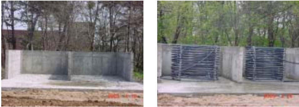
Fig. 2. Fermenting bed (left) and pipe installation (right) for hot water
