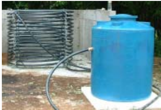
Fig. 19. Heat Exchanger System
