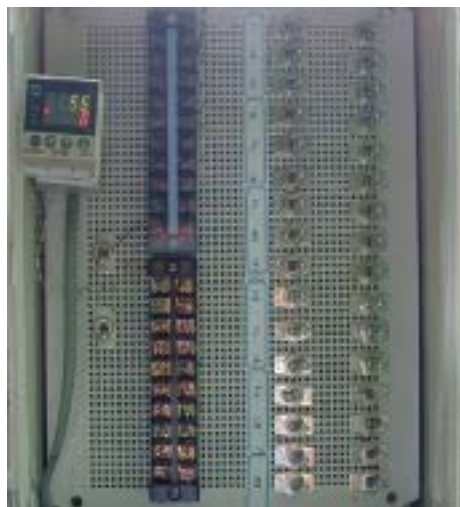
Fig. 34. Switching box (HX 4 5)
