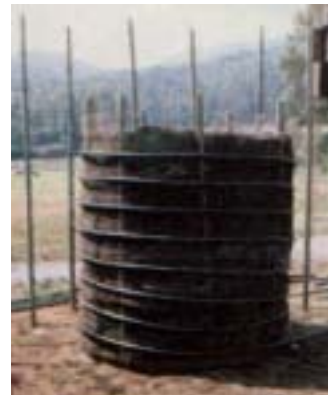
(b) Biomass Heat Exchanger interior Line
