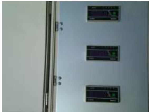
Fig. 38. Switch Box (HX 6)
