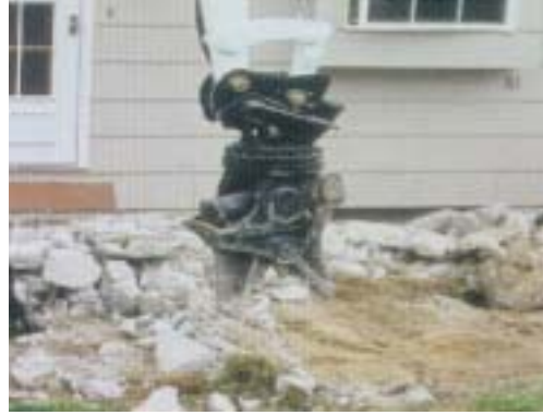
Fig. 49 View of crusher
