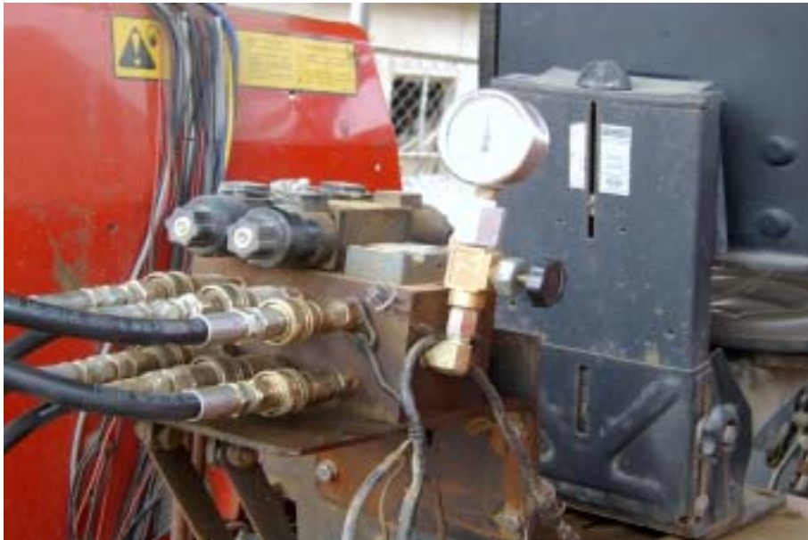
Fig. 17 View of the pressure gauge
