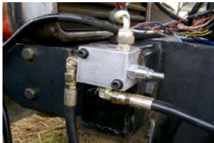
Fig. 15 View of the priority valve
